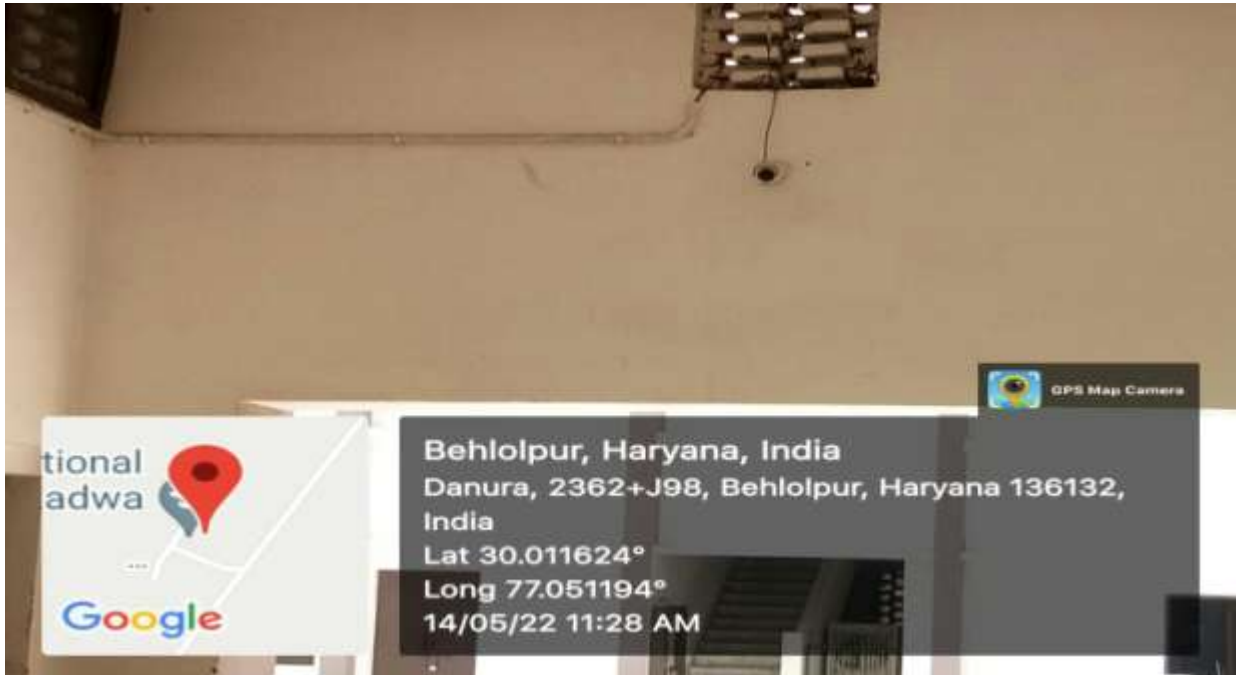
Figure 1, Surveillance Camera, Ground Floor Corridor
