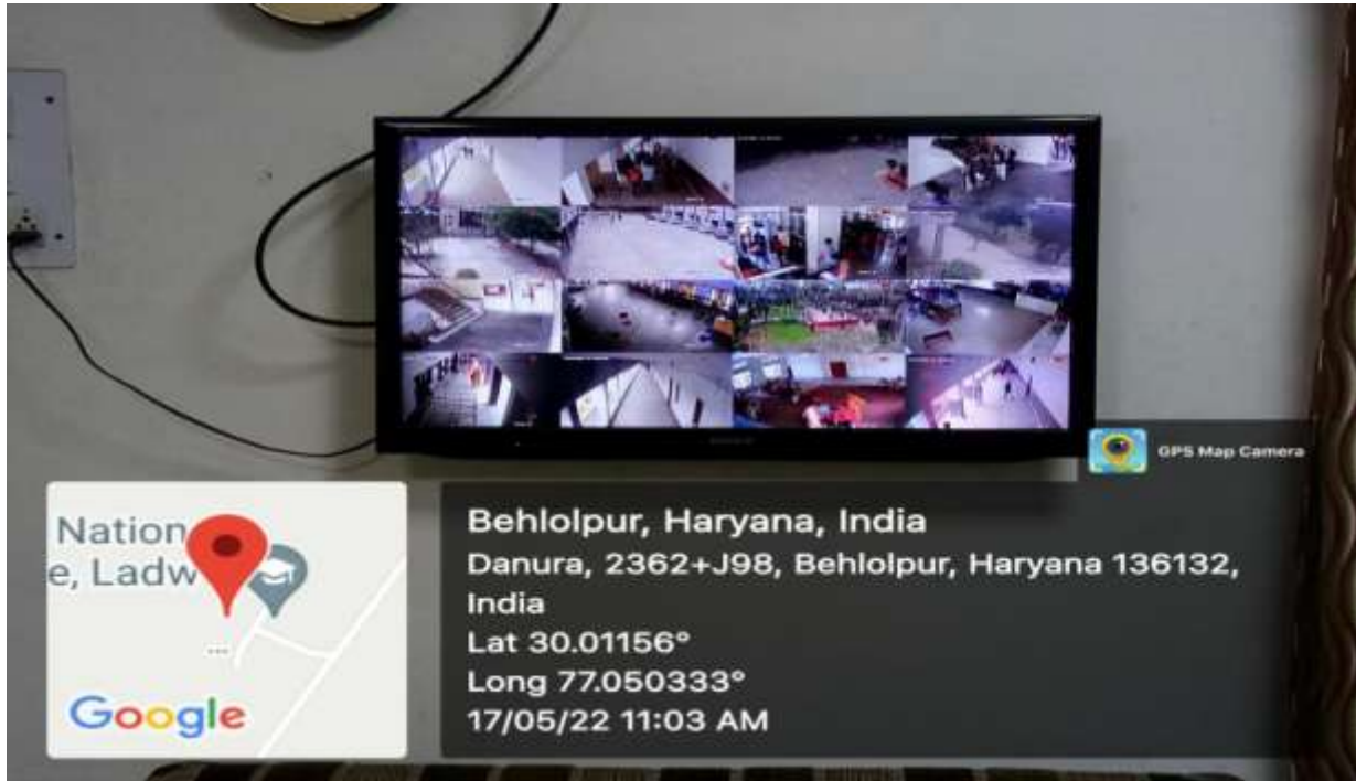
Main Screen of Surveillance System
