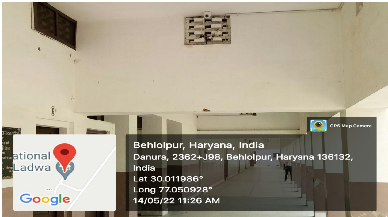
Figure 2: Surveillance Camera, Ground Floor Corridor
