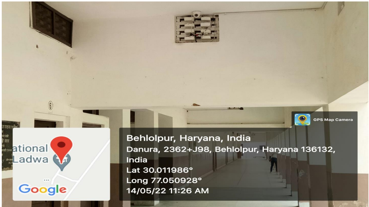
Figure 2: Surveillance Camera, Ground Floor Corridor
