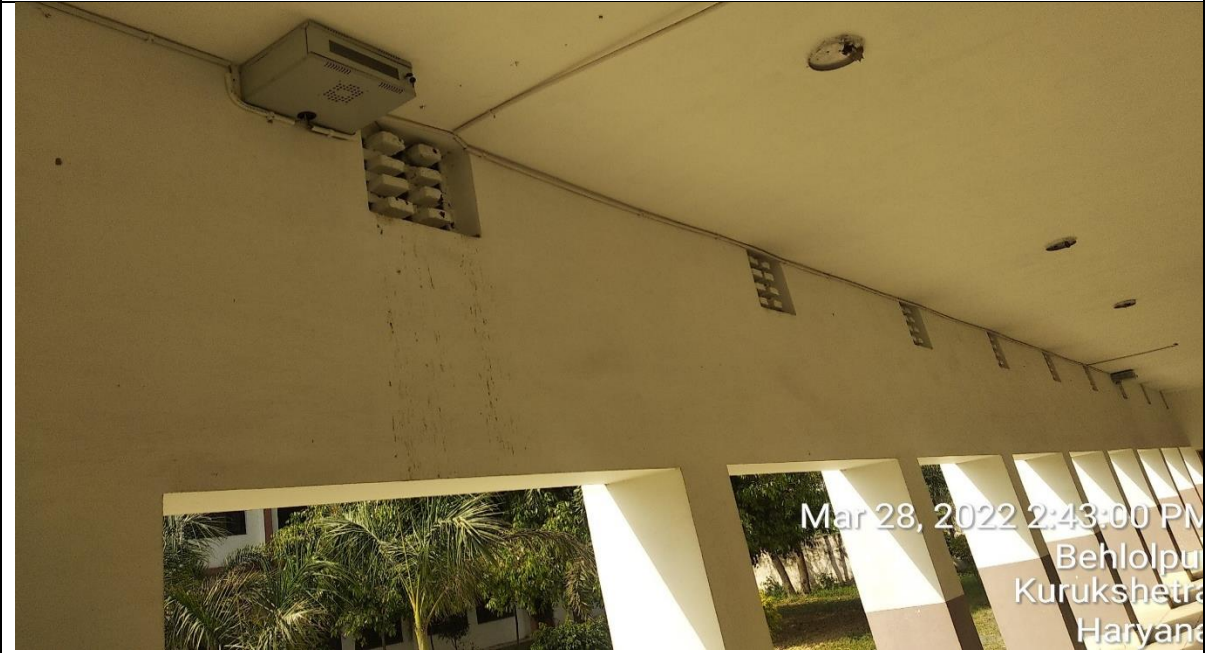
Wi-Fi Router Reck for ICT Class Rooms
