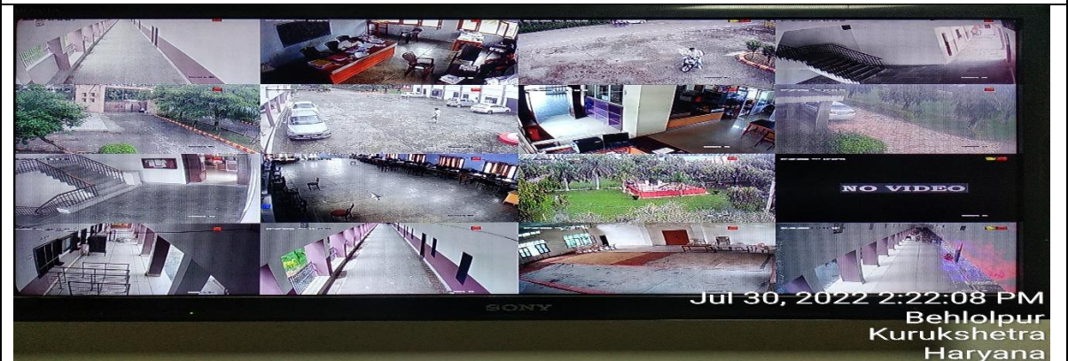
CCTV Camera's in College Premises
