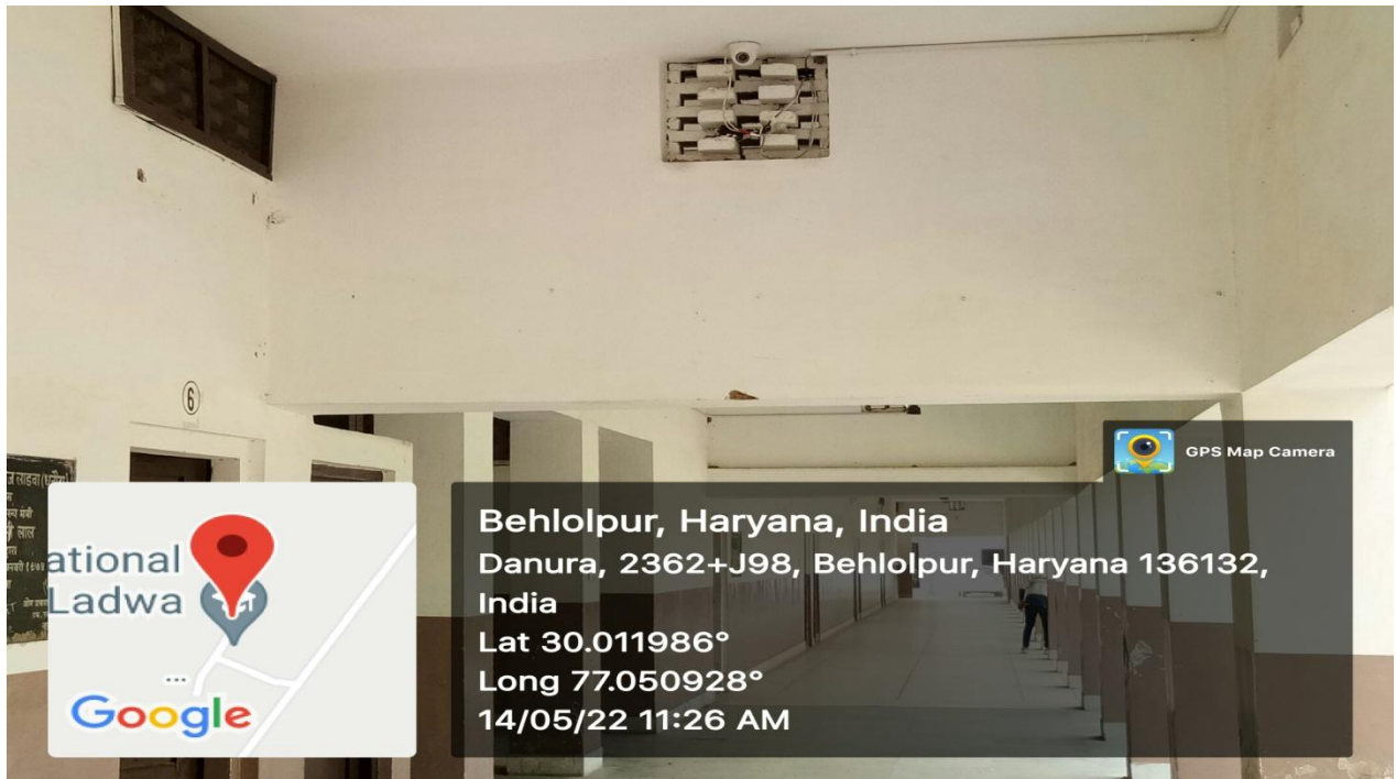
Figure 2: Surveillance Camera, Ground Floor Corridor
