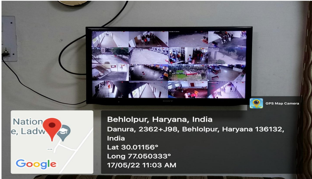
Main Screen of Surveillance System
